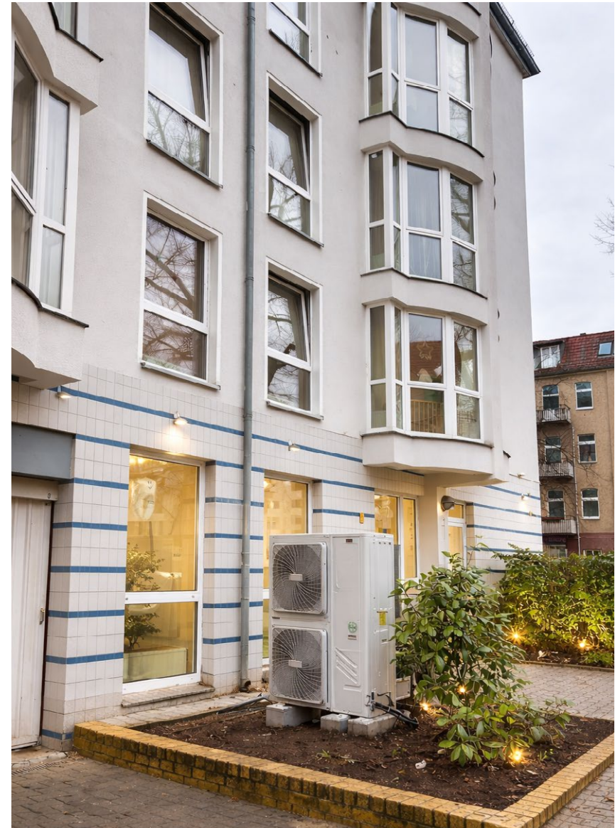
Heat pump installation at residential asset
